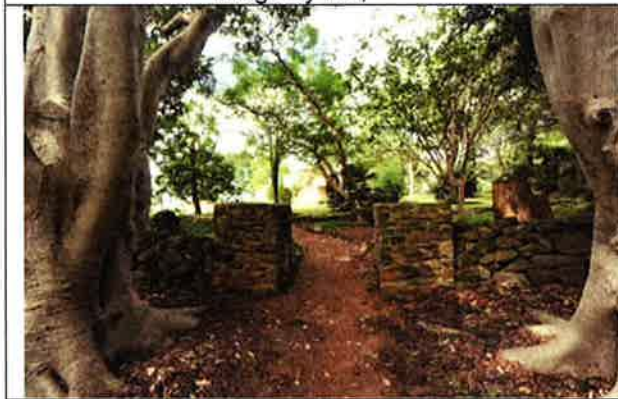
Fig. 88 The rounded wall pillars have been made square and stabilized with concrete, and the dry stone walls on each side also need correct restoration Image PD 2010
